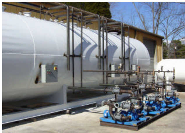
Tank with pump skid and pre-fabricated interconnect piping (prior to final painting).
