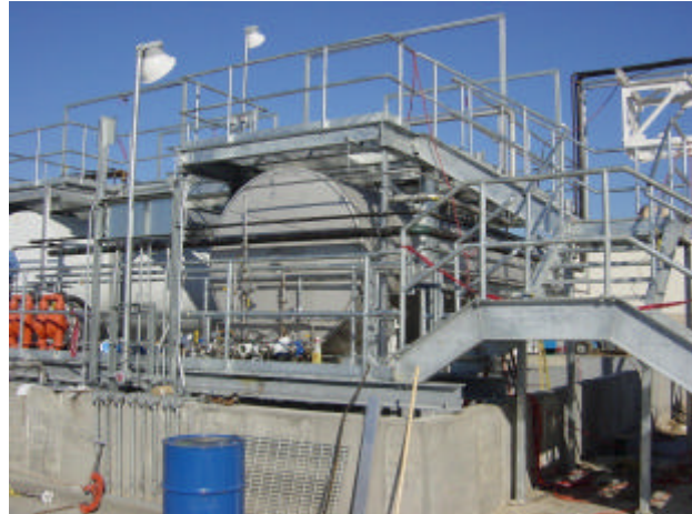
Installed 10,000 Gallon S/S brake fluid storage tank with customized pumping and instrumentation package.
