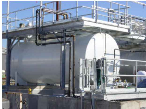
Installed 8,000 Gallon C/S methanol storage tank. All electronics and power supplies are FM Explosion-Proof certified.
