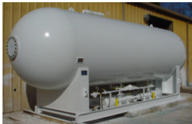
6500 gallon bulk refrigerant (R-134a) storage system.
